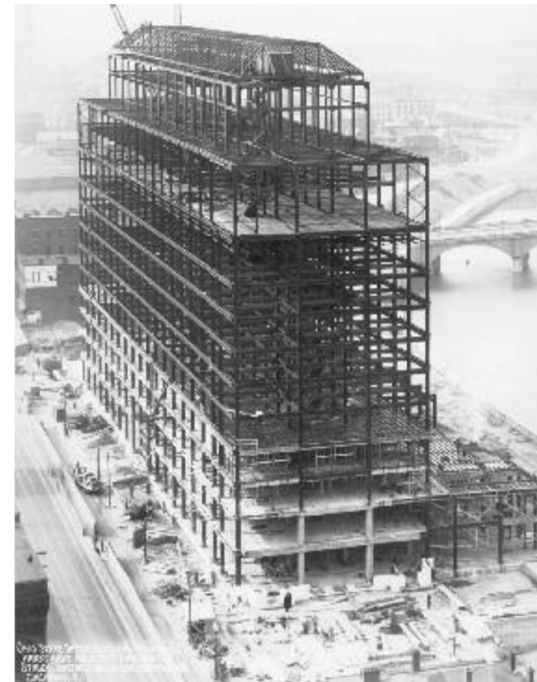
The steel frame of the State Office Building on Front Street in Columbus, May 1, 1931. The groundbreaking had taken place Nov. 19, 1929. The art deco building opened March 27, 1933, and was used for public assemblies and hearings, state offices, and the State Library of Ohio. On Feb. 17, 2004, the Supreme Court of Ohio relocated to the building and now uses it for the Supreme Court and its affiliated offices. (Ohio Historical Society)
